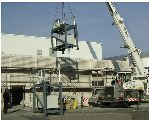
Figure 2: Linde TCF-50 Cold-box for 180 l/hr, 4.2-K LHe production (top), and Leybold vacuum pumps for 80-W, 1.8-K HoBiCaT operation being installed in the pump room (bottom).
